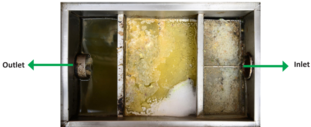
Picture: A properly maintained grease trap
