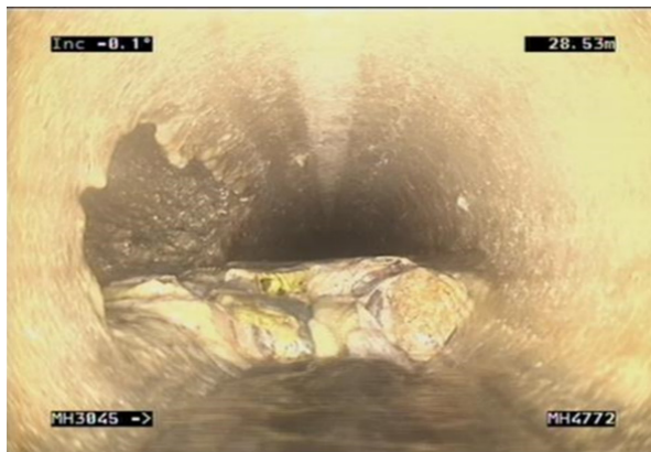
Figure: CCTV view of a wastewater pipe blocked by FOG
